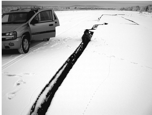
Figure 7. Fracture and lateral displacement of the northern end of the runway at Northway Airport (near SASW Site 582-NOR and 587-NOR). Fissures formed along the pavement seams of the runway.
